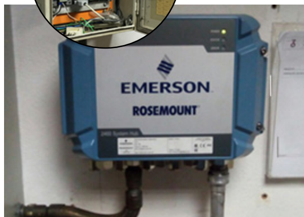
After: Newly installed Rosemount 2460
